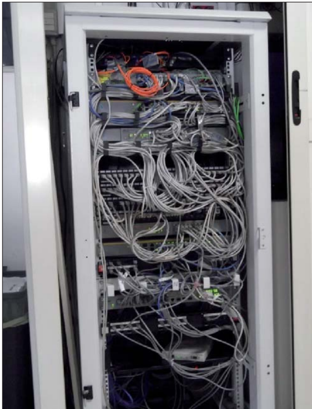
"Armandi" contenenti switches e routes
